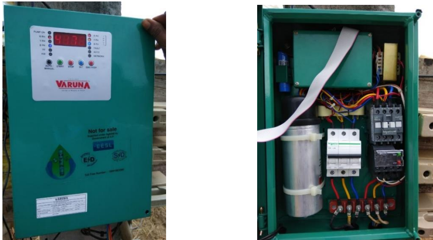
Figure 28: Smart Control Panels distributed in AgDSM in Andhra Pradesh
