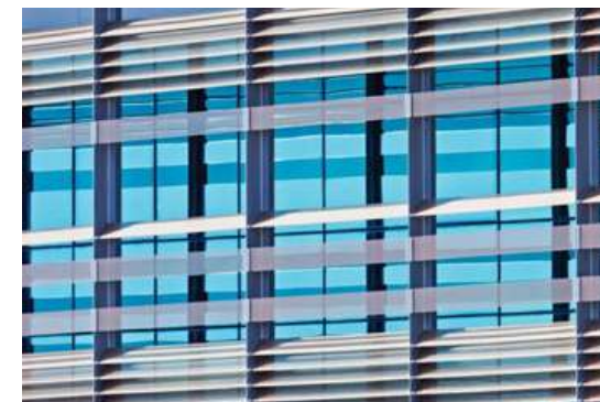
FIGURE 18 AUTOMATED SHADING DEVICES
