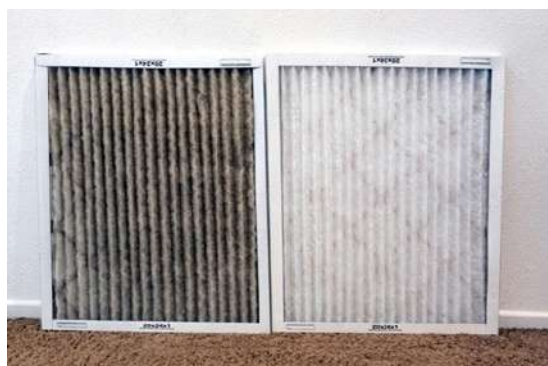
FIGURE 27 AIR FILTER MAINTENANCE
