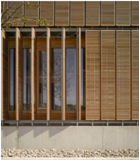
FIGURE 19 AUTOMATED SHADING SYSTEMS
