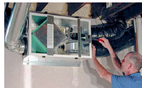
FIGURE 37 ENERGY RECOVERY VENTILATION SYSTEMS
