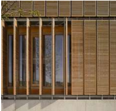
FIGURE 28 AUTOMATED SHADING SYSTEMS
