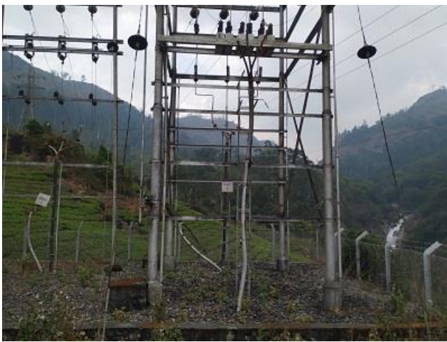
Switching station yard
