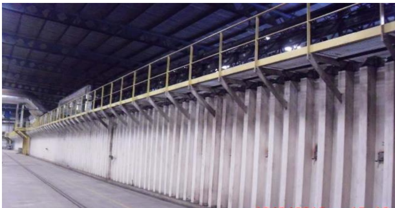
Fig Tunnel kiln
