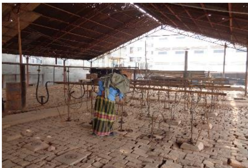
Figure 14 Use of Natural Gas in a Hoffmann Kiln in Bangladesh (Source: GKSPL)
