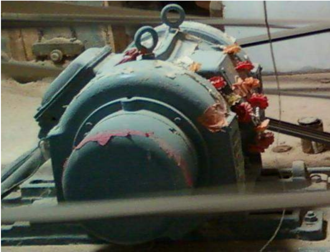
Figure 12: Old and Rewinded Inefficient motor
