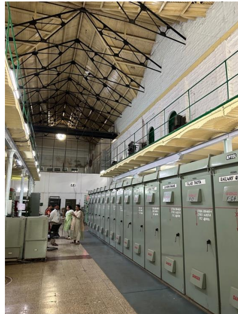
66 kV Substation Control Room
