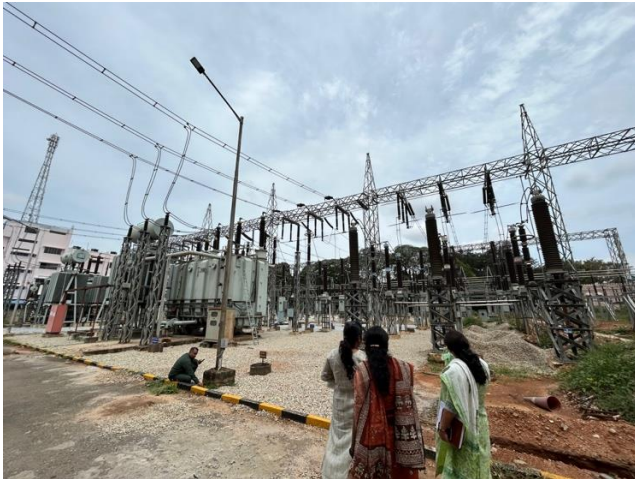
KPTCL 220 kV Substation Yard
