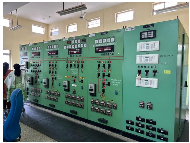
KPTCL 220 kV Substation Control Room
