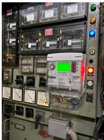
11kV Metering Bank
