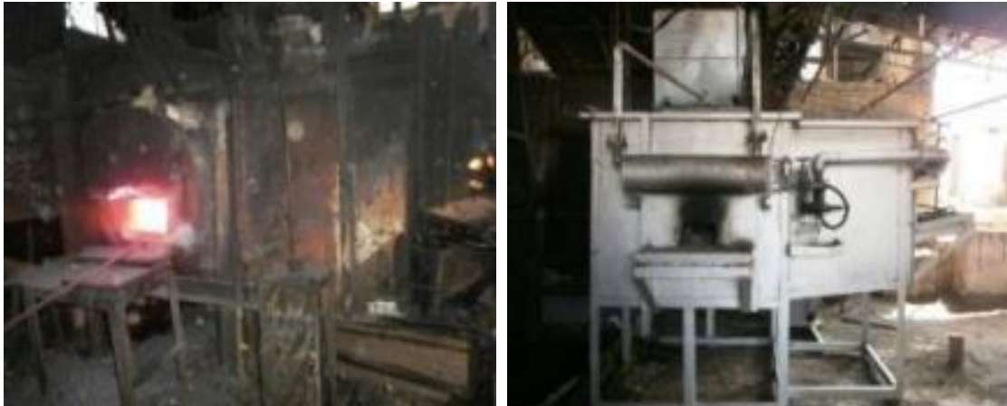
Inefficient Forging Furnace
