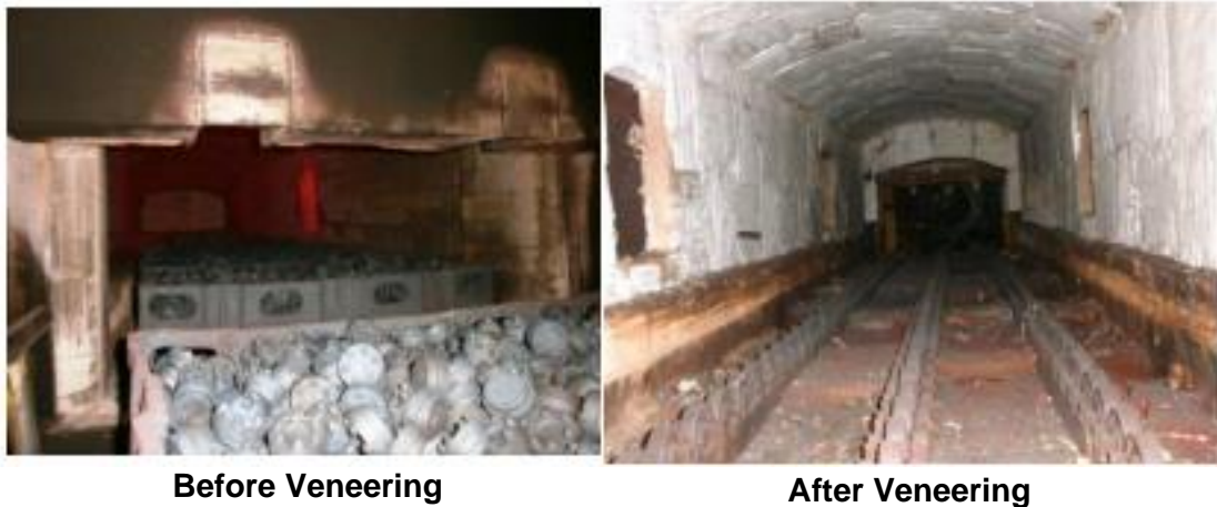
Figure 26: Application of veneering module in LPG Fired Normalizing Furnace
