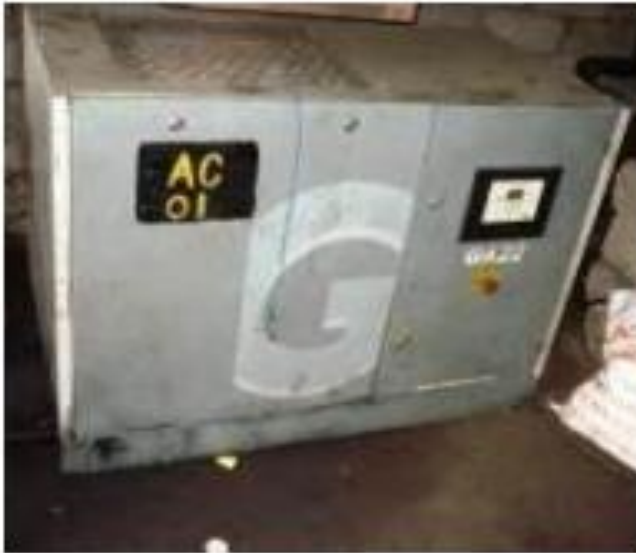
Existing Air Compressor
