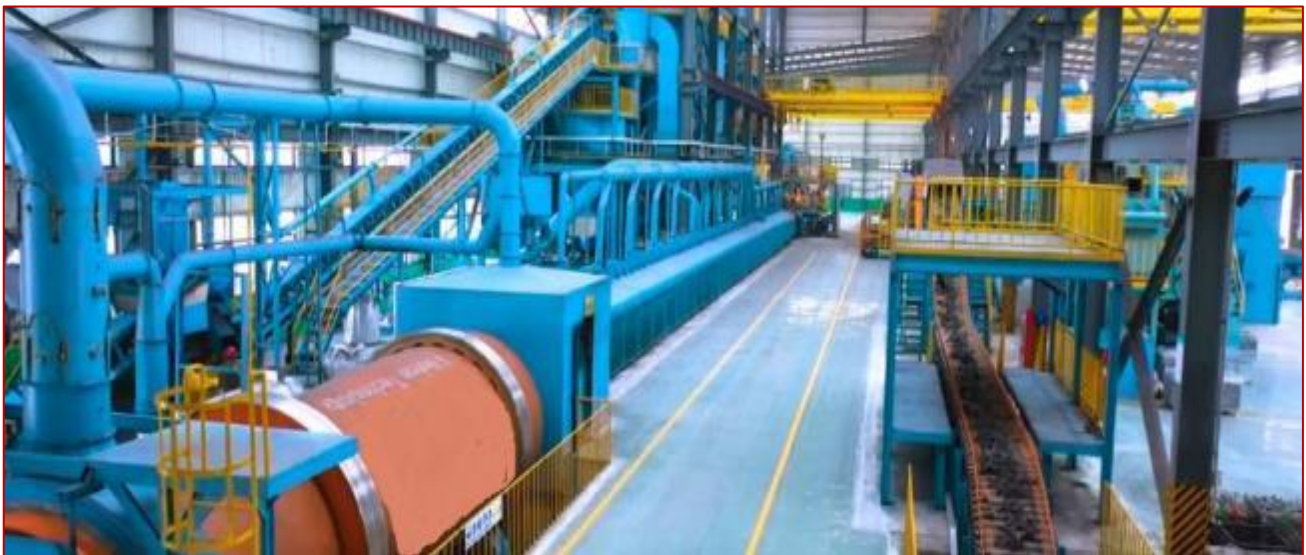
Figure 51: Integrated Sand plant with automation 67
