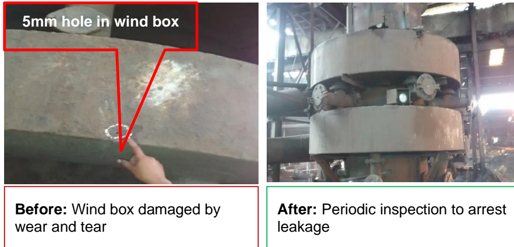
Figure 72 Air leakage in wind box
