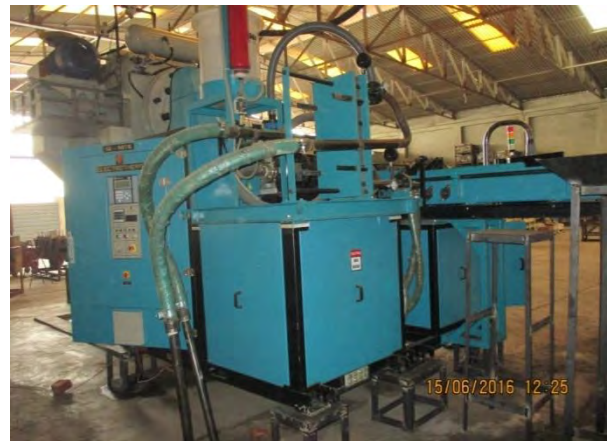
Figure 2.6: Induction heater of capacity 200 kW installed at Global Exports India
