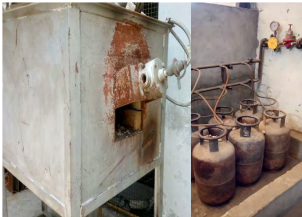
Figure 2.5: Snap shot of LPG based re-heating furnace at Global Exports India (operational during baseline)
