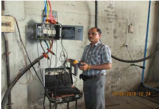
Figure 2.3: Post implementation energy audit at Global Exports India
