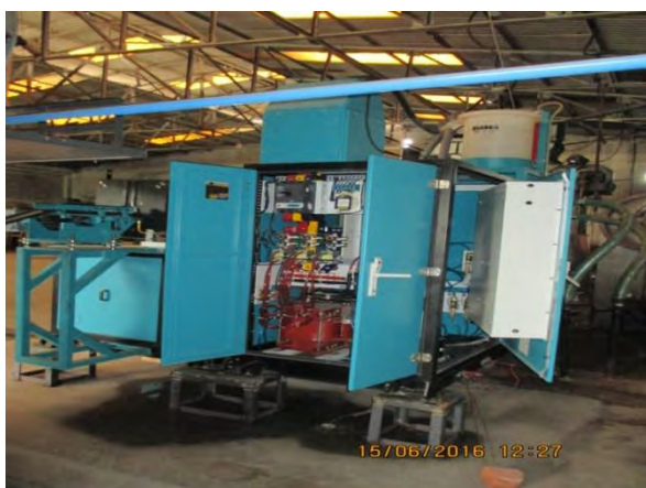
New Induction heater installed of capacity 200kW at Global Exports India
