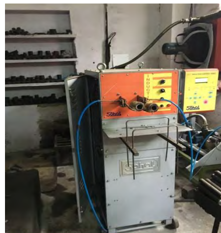
Figure 2.5: Induction heater of capacity 30kW installed at NN Products (India)
