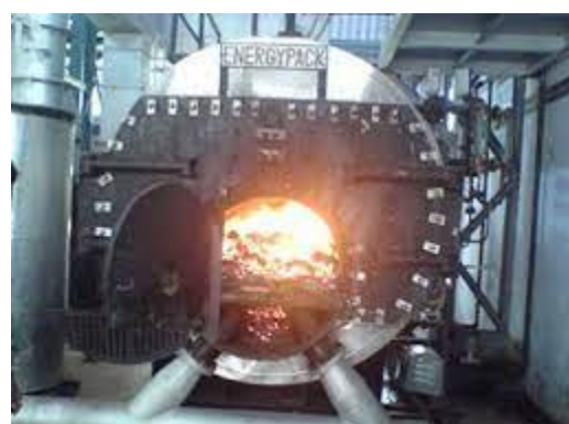
Figure 114: Biomass boiler and wood pellet fuel
