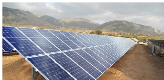
Figure 107 Solar PV plant
