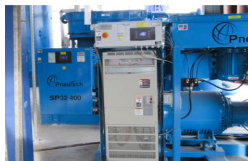
Figure 95: VFD Air compressor
