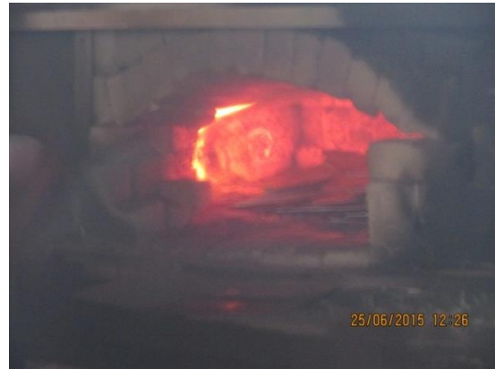
Snap shot installed FO based re-heating furnace at Saggu Toka Industries (presently not in use)
