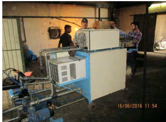
Figure 2.6: Induction heater of capacity 100kW installed at Saggu Toka Industries
