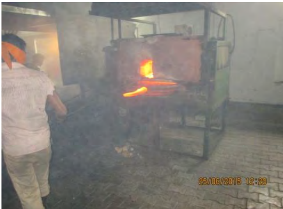
Figure 2.5: Snap shot installed FO based re-heating furnace at Saggu Toka Industries (presently not in use)
