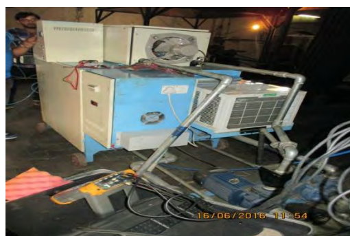
Figure 2.4: Post implementation energy audit at Saggu Toka Industries
