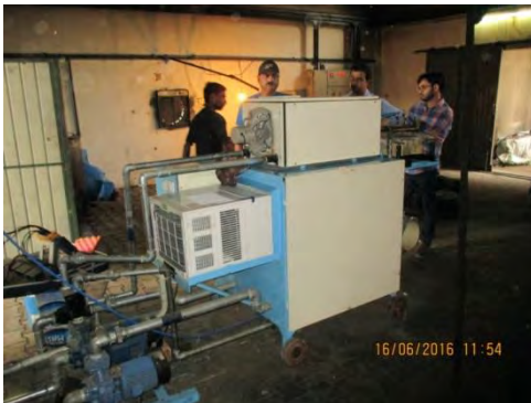
Induction heater of capacity 100kW installed at Saggu Toka Industries
