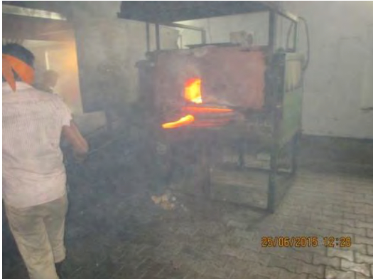
Snap shot installed FO based re-heating furnace at Saggu Toka Industries (presently not in use)
