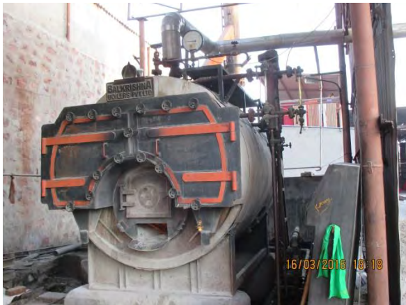
Caption: Boiler unit at Shree Rajaram Process
