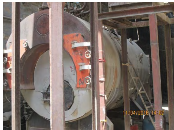
Caption: Boiler unit at Sonu Industries
