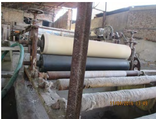
Caption: Caustic processing unit at Sonu Industries
