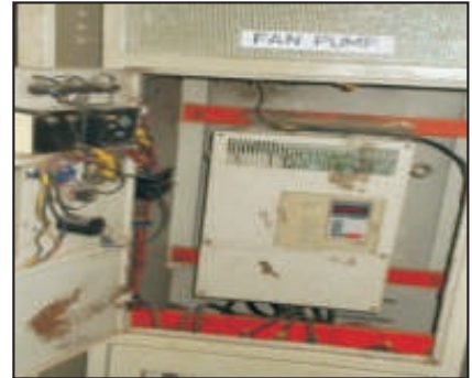
VFD Control Panel on Fan Pump 100 HP
