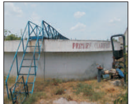
ETP system for water recovery
