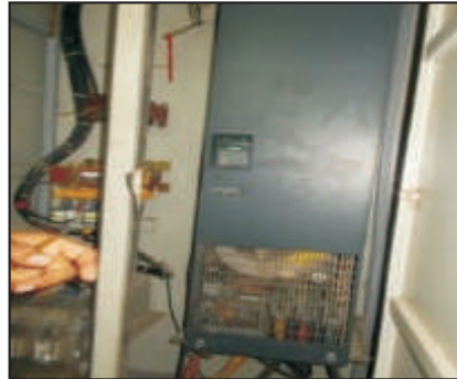
VFD Control Panel on 150 HP Vertical Pulper Motor
