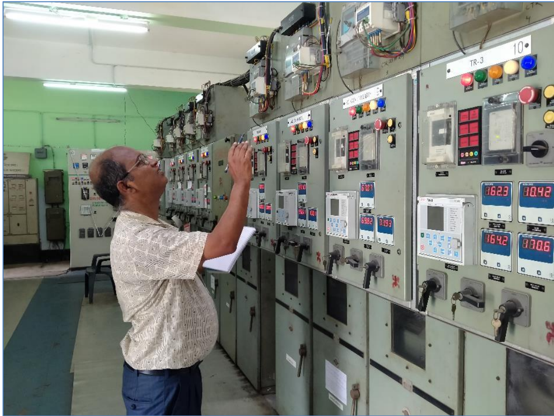
Figure: Verification of Energy Meters at M-III Substation
