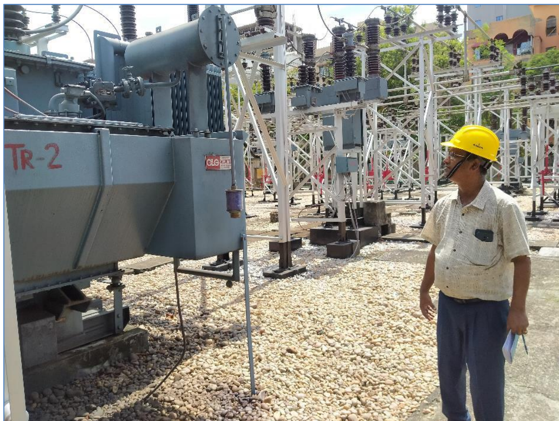
Figure: Visit at M-III Substation
