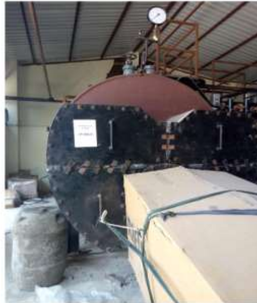
New 4 TPH Boiler at OMFED, Bhubaneswar
