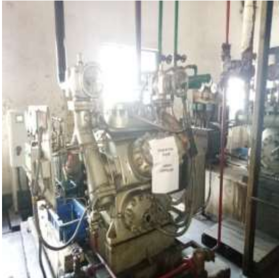
New Ammonia Compressor at OMFED, Bhubaneswar
